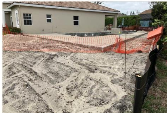
Rear view of pool and deck construction progress. North/rear fence will run along the rear property line (N 61°09' E - 75.53').
