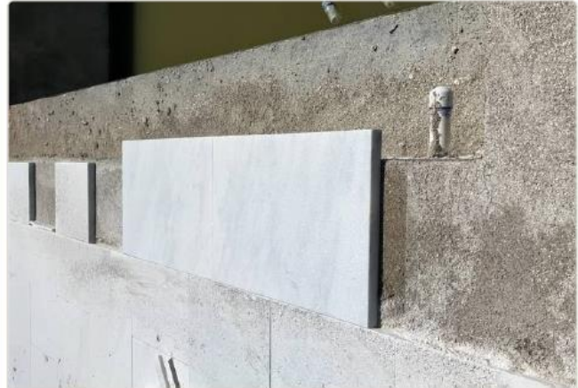
Aurora Sandblasted Marble coping close-up — deck and pool coping material used throughout 865 SF deck area.
