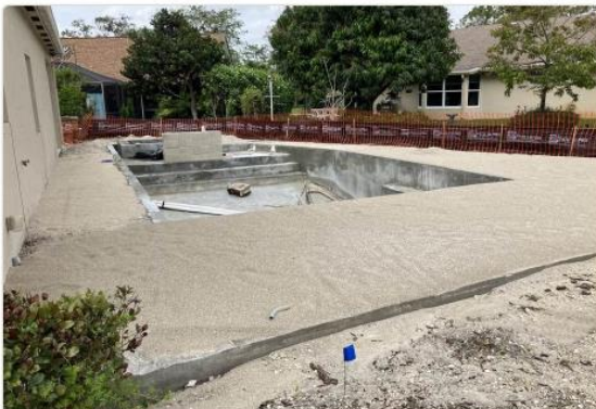
Pool shell construction in progress. Shows pool position north of house relative to property boundaries. Fence will enclose this area along north and east property lines.
