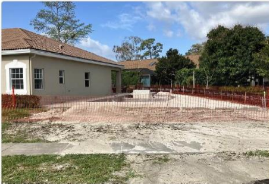
14596 Horseshoe Trace — street view during pool construction. Shows property frontage on Horseshoe Trace (east), house, and construction area. Fence will be installed following pool completion.
