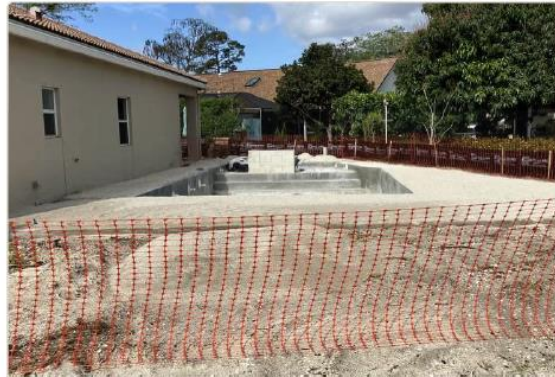
14596 Horseshoe Trace — side view showing pool construction progress and property layout. North side of house visible.
