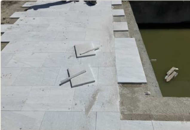
Aurora Sandblasted Marble deck installation — top view showing deck surface material and layout. Fence posts will be surface-mounted through existing pavers.
