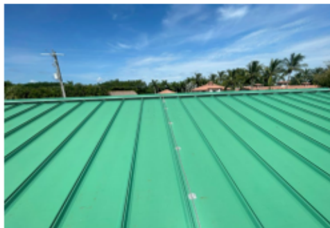
LP on roof
