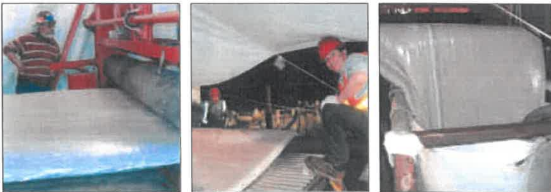
"Over the hole" wet out and installation of large bore circular, non-circular, and box culvert applications
